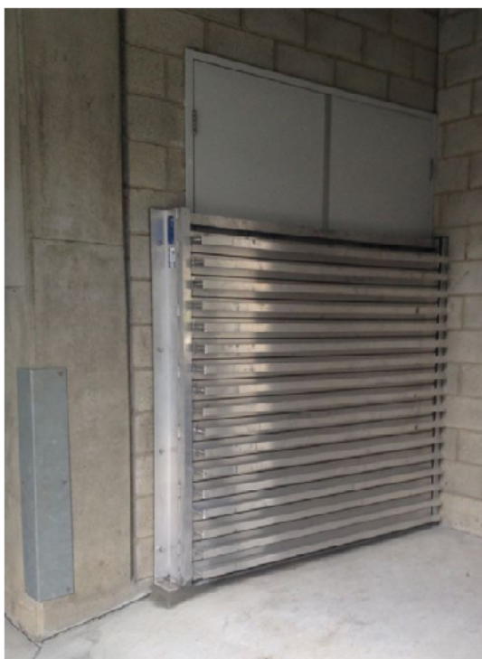
Figure 62: A retrofit example of manually installed segmented flood barriers to protect building services during flood events.
