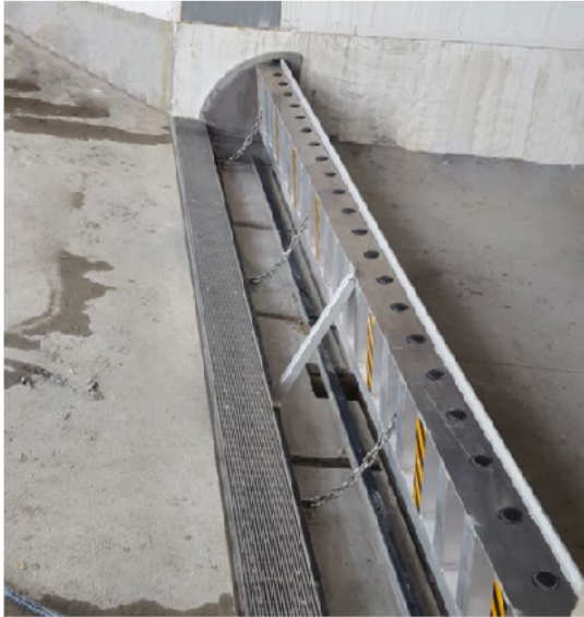
Figure 68: A self-actuating tilting flood barrier protects the entrance to a basement.
