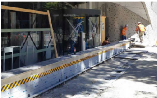
Figure 72: The barrier is concealed beneath the pavement with a top plate, side panels and drainage system integrated into the paving.
