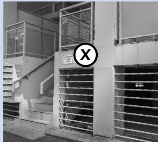
Figure 60: The interface must be carefully designed to ensure a positive relationship to the street. This example shows a raised ground floor to allow for water to flow underneath the building. It has resulted in a dark enclosed space at street level that regularly gets filled with rubbish.
