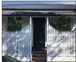
EX.001 GALVANISED IRON ROOF SHEETING (AS PER ORIGINAL) FINISH: PAINTED DARK GREY AS PER ORIGINAL LOCATION: FRONT TRANSVERSE GABLED ROOF + VERANDAH BULLNOSE ROOF
