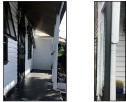
EX.005 REINSTATED TIMBER VERANDAH POSTS FINISH: PAINTED AS PER ORIGINAL LOCATION: FRONT FACADE VERANDAH
