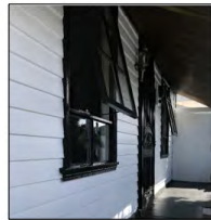
EX.004 REINSTATED ORIGINAL WINDOWS WITH SIMPLE ARCHITRAVE SURROUND FINISH: PAINTED AS PER ORIGINAL LOCATION: FRONT FACADE
