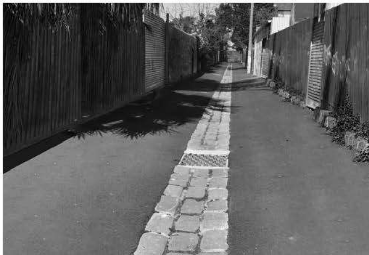
Photo 22. This laneway in St Kilda has been sympathetically re-constructed to retain the traditional blue stone channel and a asphalt surface.
