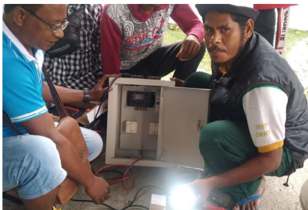
The CCC team installed solar lighting in sacred houses as part of a UNDP funded project
