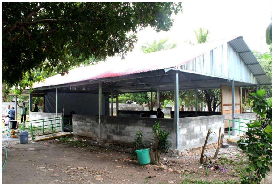
The CCC training room was rebuilt due to flood damage and is now hired regularly by community groups.
