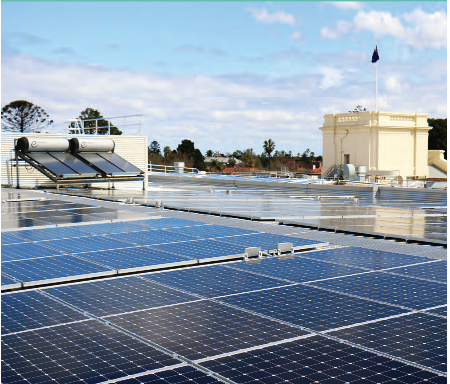
Solar panels on the St Kilda Town Hall roof
