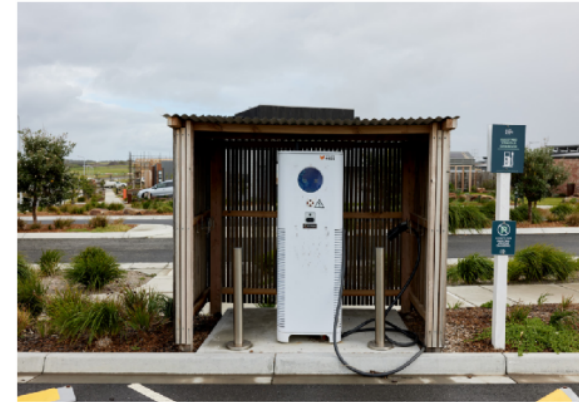
Electric vehicle charging station at The Cape development. Photography by Kim Landy
