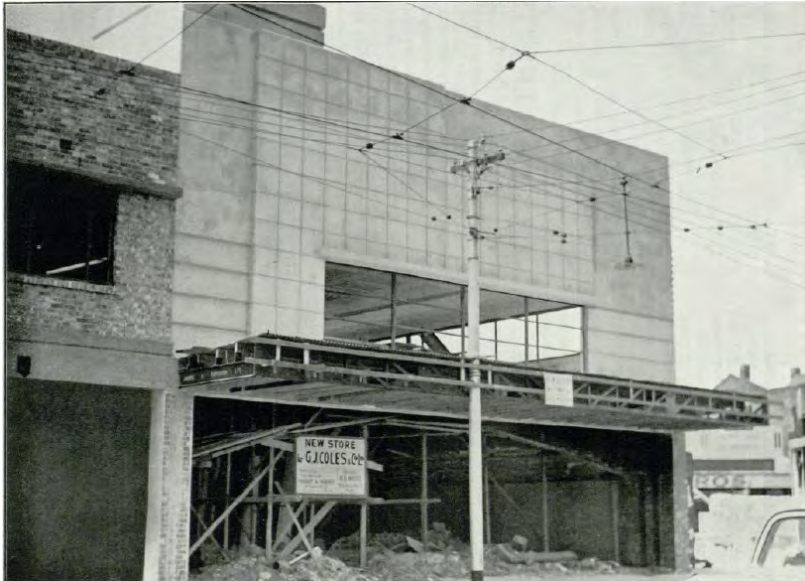
Figure 21 – Shows two buildings under construction in 1938, the Coles store at 156-160 Acland Street, as well as the building to left, part of the St Kilda Market site (now 181-89 Barkly Street). (Source: Colesanco 1938 , vol. 10, issue 47)
