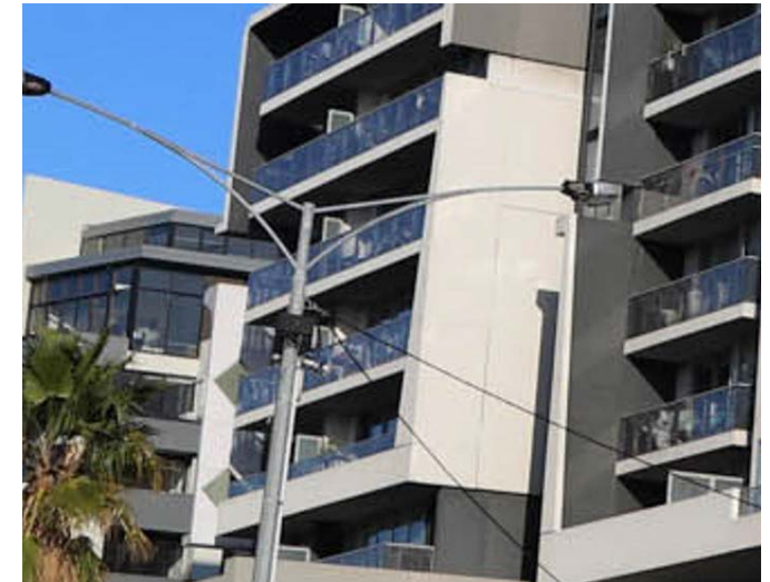
Heavy framing elements to balconies diminish upper level setback objectives
