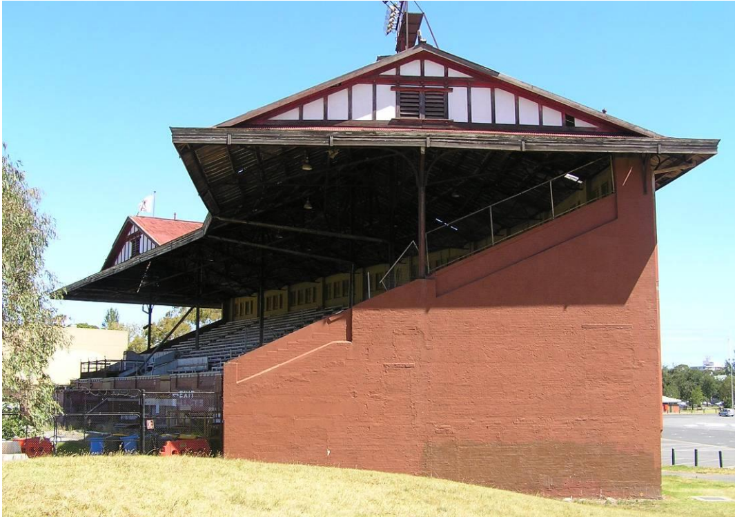
Figure 6.38-8 – The South Melbourne Cricket and Football Club Grandstand, (1926-28) showing distinctive cranked form and open roof carried over trusses with gable ends.
