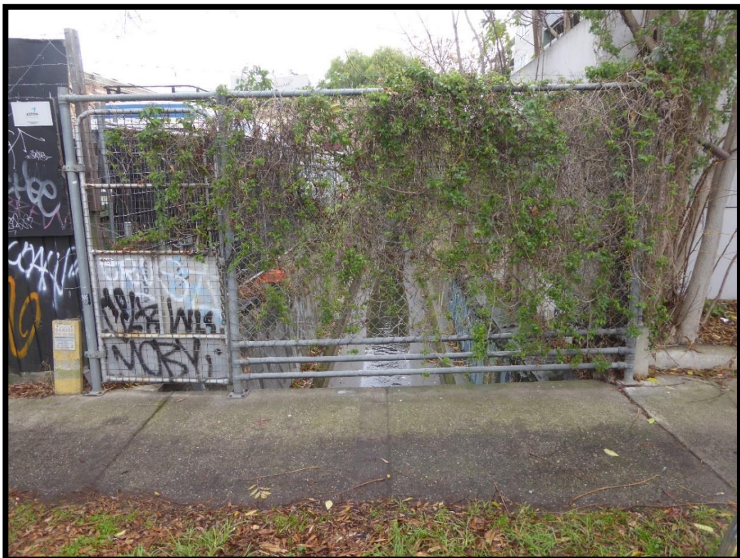
Greeves Street West cyclone fence barrier and gate W.4000 x H.2110mm.
